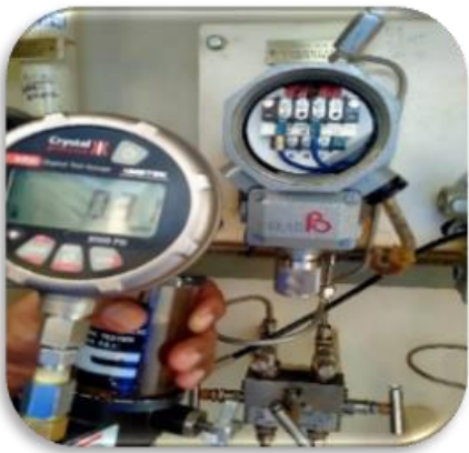
Gambar 7. Pengujian Differential Pressure Switch
